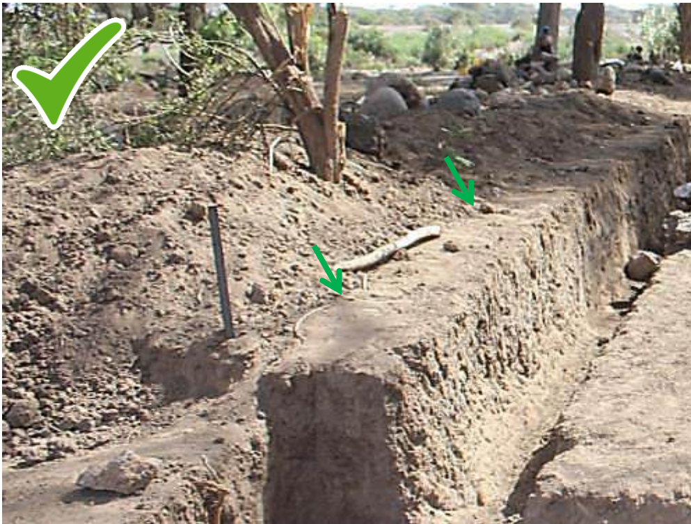
አፈሩን ከጉድጓዱ አርቆ ማስቀመጥ:: Soil is placed far away from the excavation.
