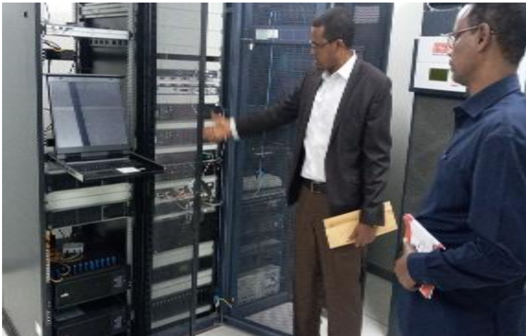
Figure 4. Data center at BoIT
