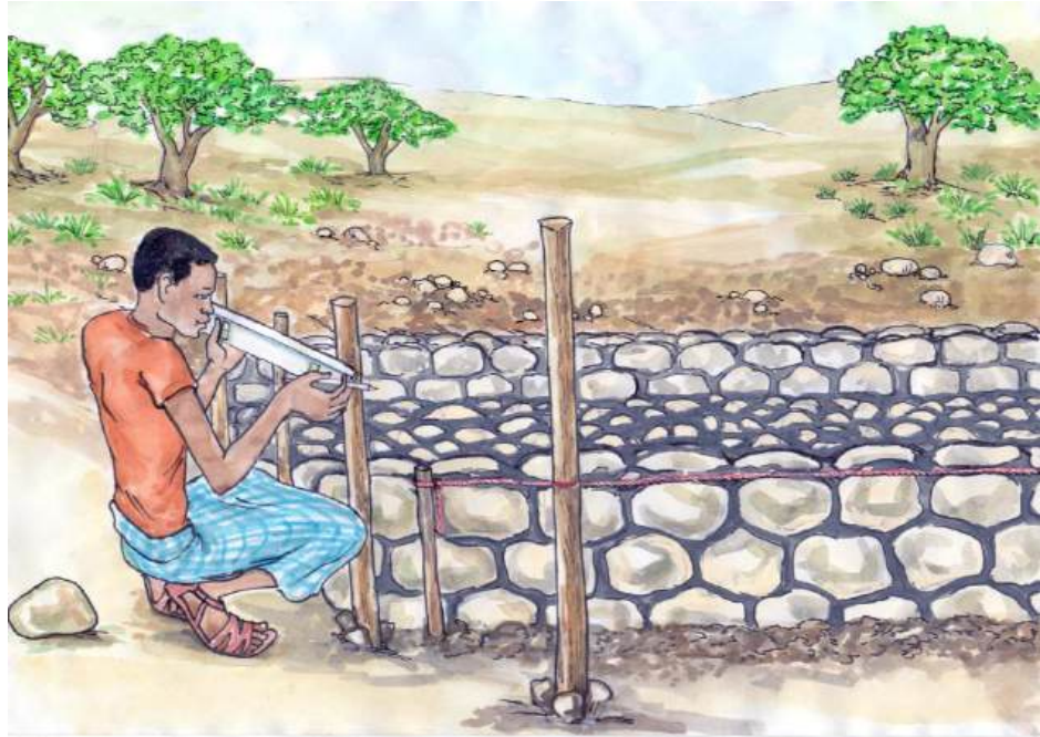
Illustration 45: the DA checks on the newly constructed part using the spirit level.
