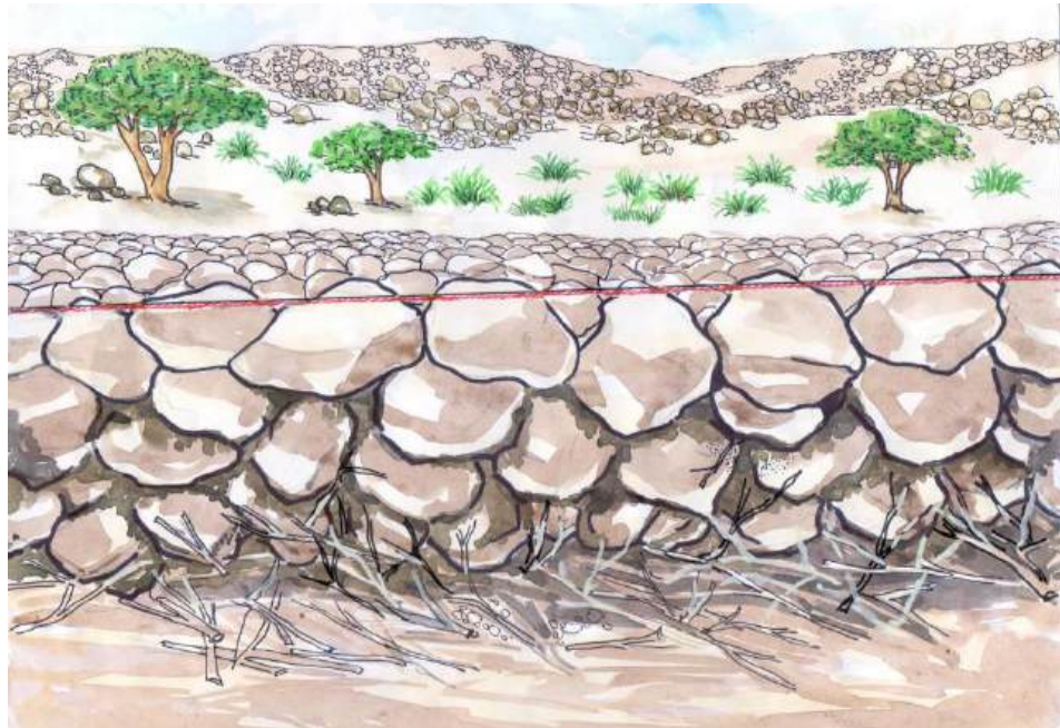
Illustration 18: The construction seen from upstream. The wall made of big stones, the rope demarcating the upper straight line of the dam. Small stones in the back indicate that the construction is not yet finished. A cover layer of big stones is missing.
