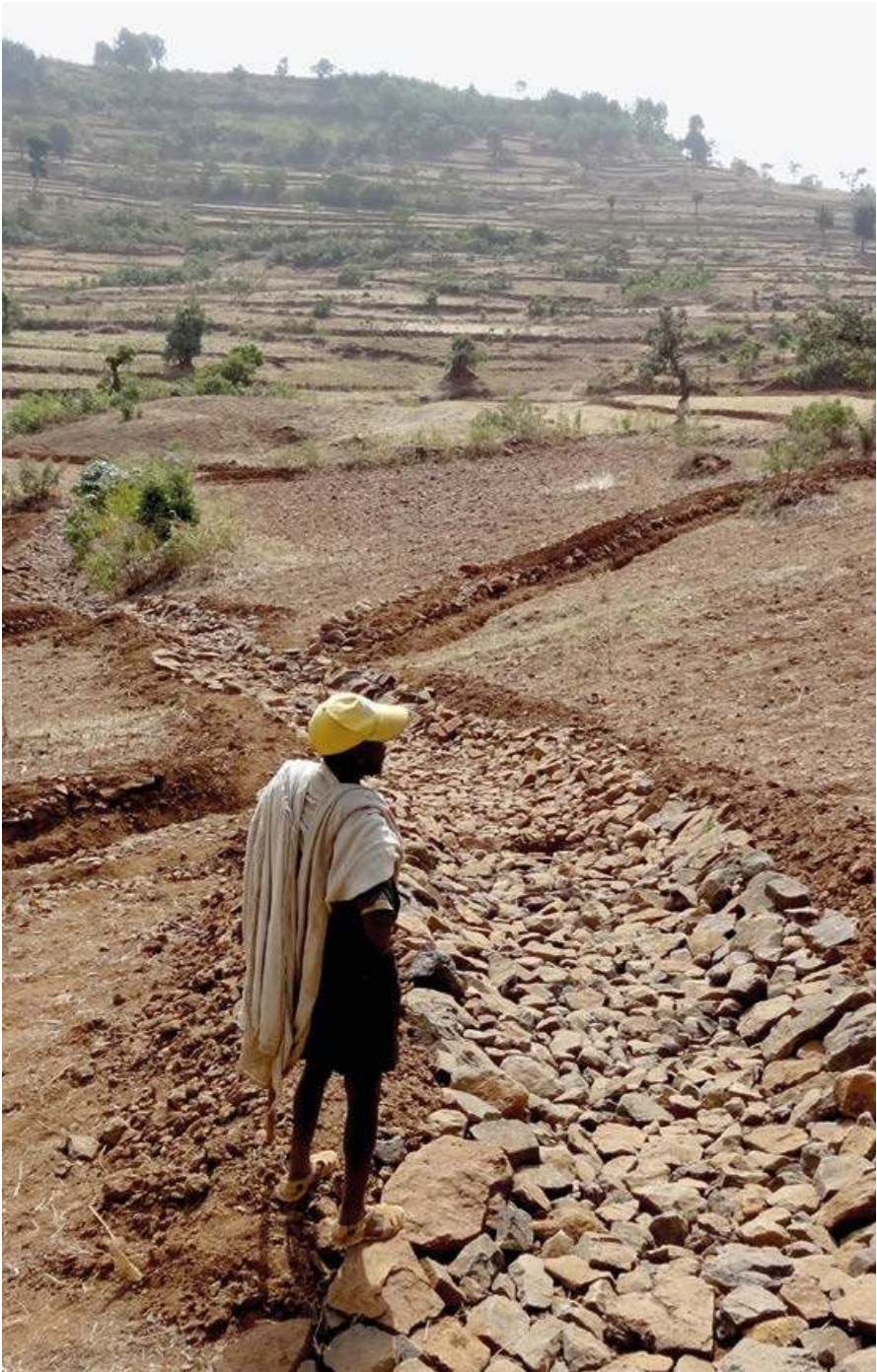
Stone-paved Cutoff Drain in Abagerima area, South Gonder (2013).
