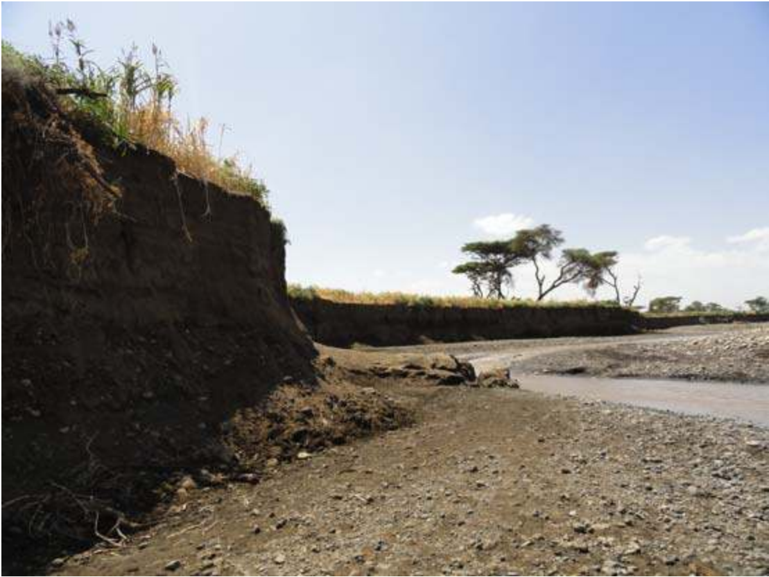
Figure 5 – Stream-bank Erosion in Hida
