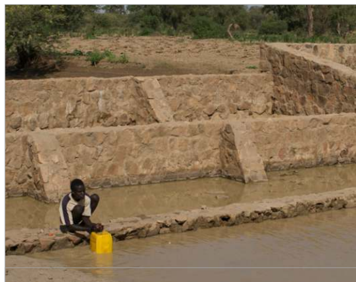
Stagnant water in water-spreading weir
